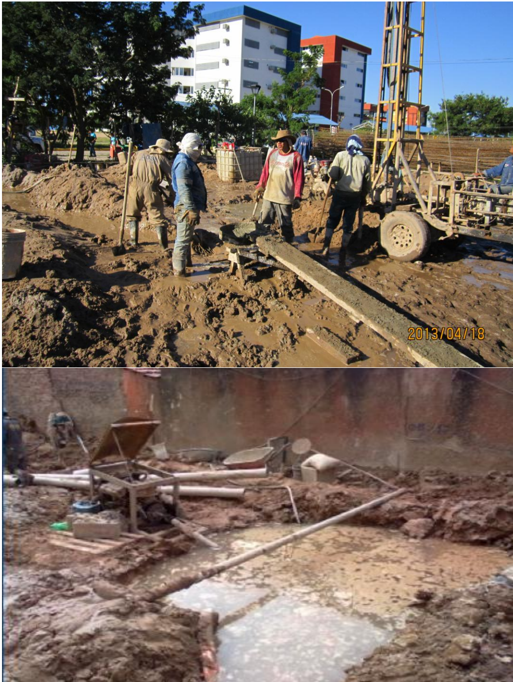
Fig. 2 Photos from a construction site in Santa Cruz, Bolivia, showing rig and collection pit
